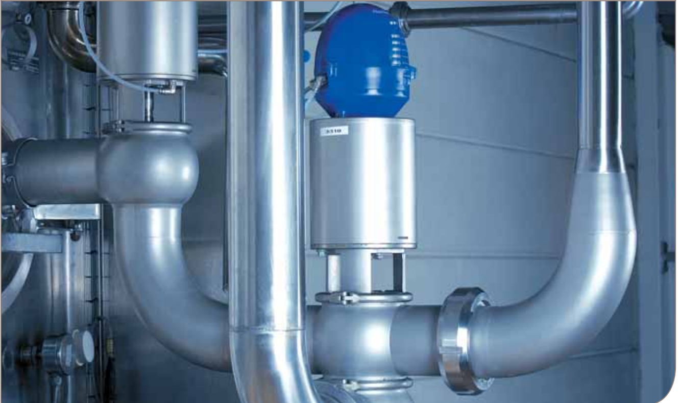
Unique 7000s installed in the Christiansfeld dairy.
